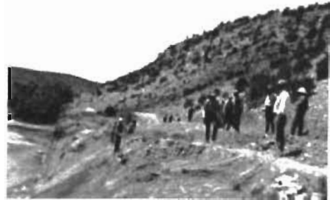
Works Progress Administration employees digging new irrigation ditch and moving road above Villanueva after the record floods of 1937. Photograph courtesy of New Mexico State University Archives Photographic Collections.
